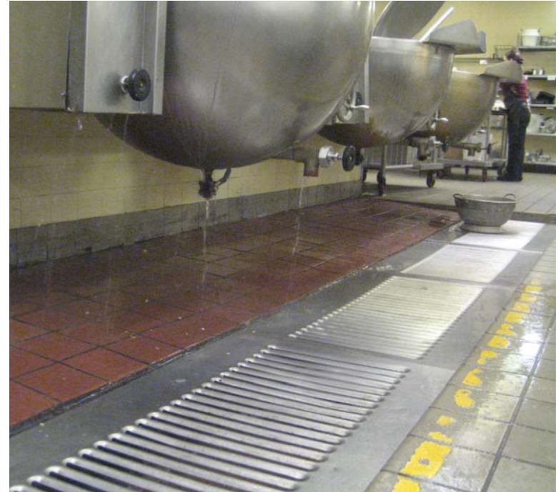
P1: Trench drains
