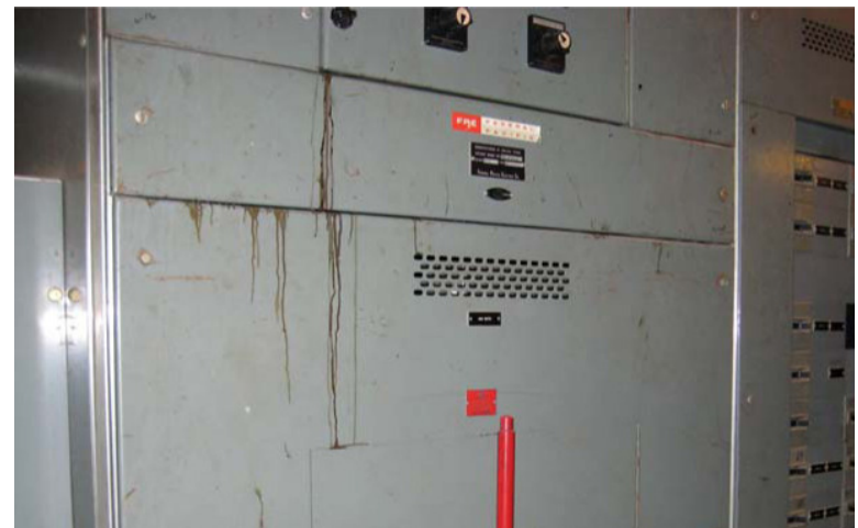
E2: Main Switchboard Main Disconnecting Means
