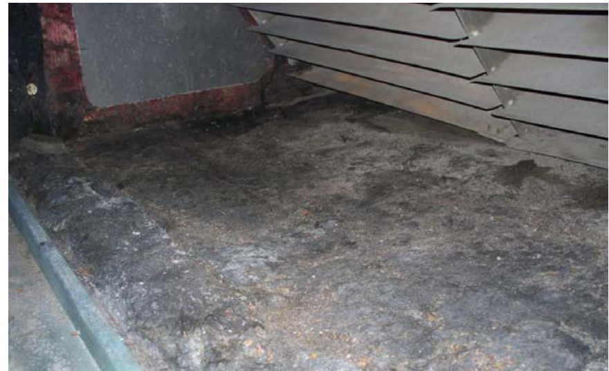
M1: Fraying ductliner
