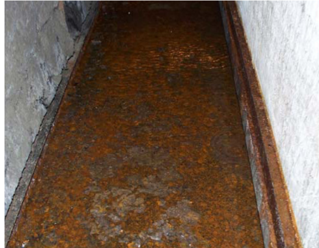
M2: Rusting drain pans and coil casing
