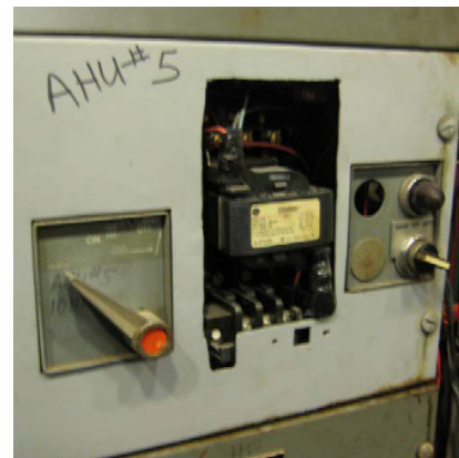
Modified Federal Pacific Motor Control Center Bucket
