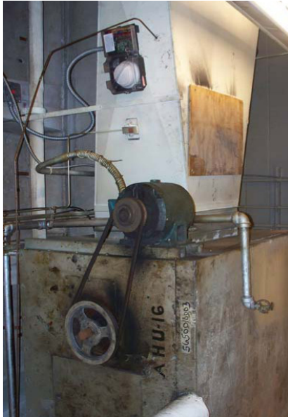
M3: AHU Motor with no belt guard
