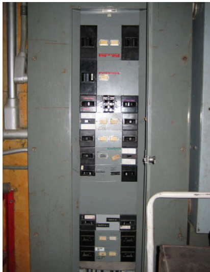
E15: Overall picture showing emergency distribution panelboard EDP.
