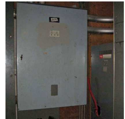
E14: LakeShore ATS case with ASCO transfer switch components installed.
