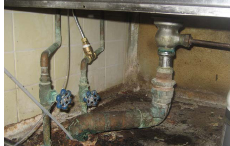
P2: Drains below sinks
