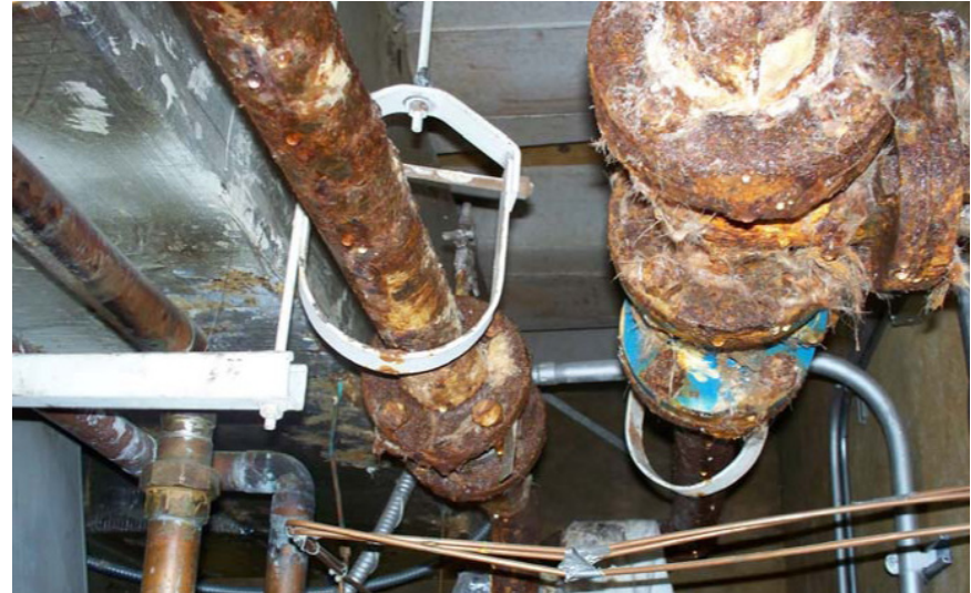
M5: Hot Water Piping
