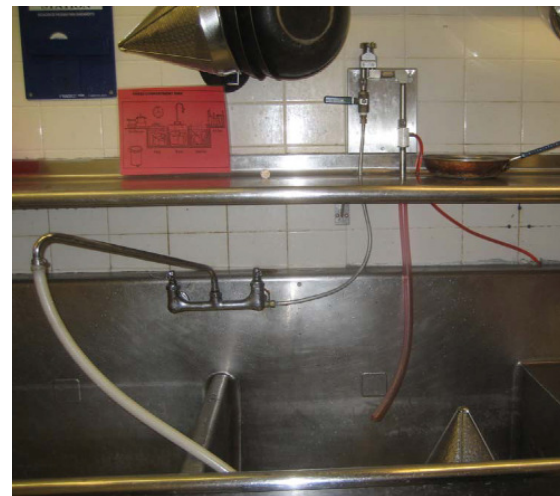
P3: Hoses extending below the level of the sink edge
