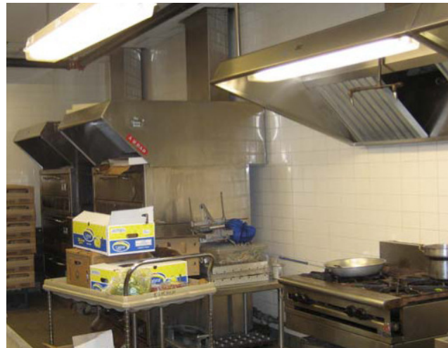
M4: Kitchen Exhaust System
